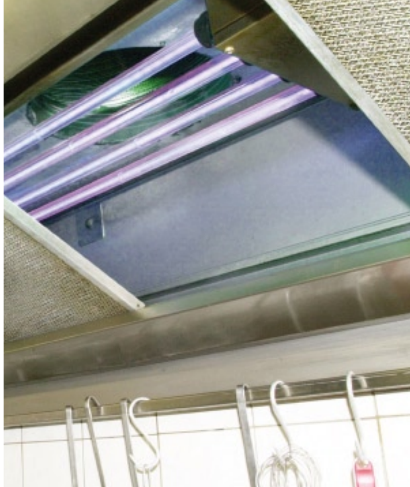
“Cold burn-off” of greases in a kitchen hood
